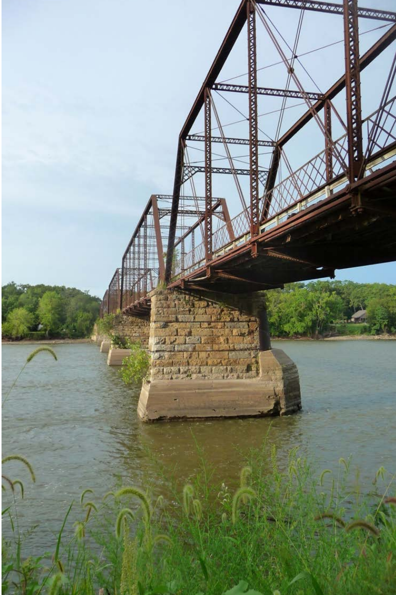
Rehabilitation of the Bentonsport Bridge, a pedestrian bridge, is one of the new Great Places projects. (Courtesy of the Bentonsport Improvement Association)
